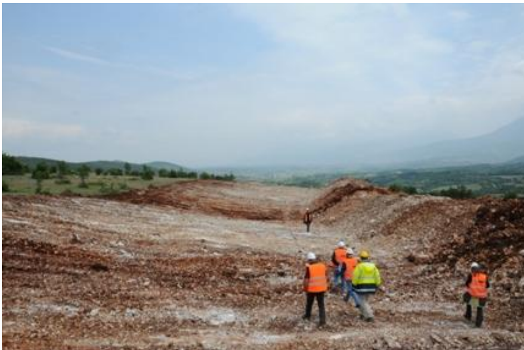
Photo 6 – Ripped Material from Alignment
